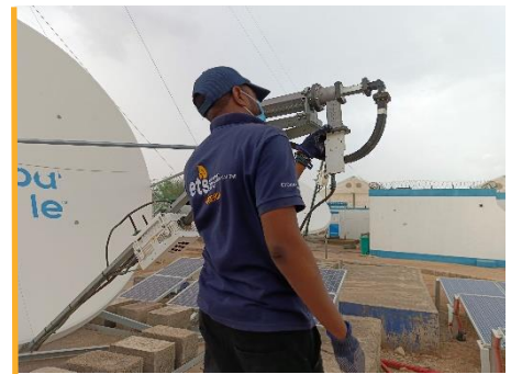
The ETS conducts routine maintenance on the internet infrastructure in Banki. Photo: WFP/ETS
