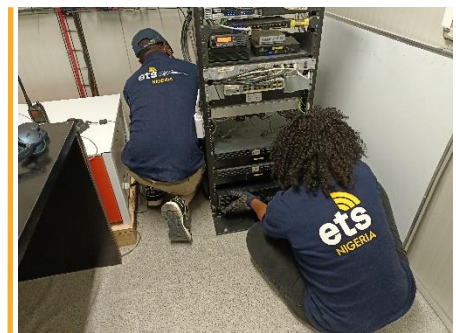
The ETS installed new Uninterruptible Power Supply (UPS) devices in Damasak. Photo: WFP/ETS
