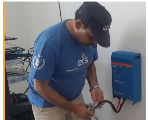
ETS staff installs solar power equipment in the security communications centre in Dikwa. Photo: WFP/ETS
