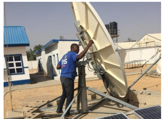
An ETS staff member conducting a satellite site survey in Damasak humanitarian hub.
