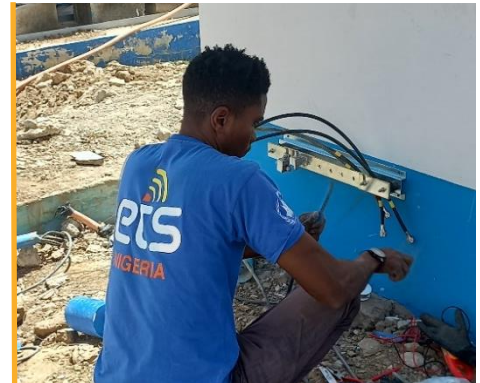
ETS staff connecting security communications equipment in Dikwa. Photo: WFP/ETS
