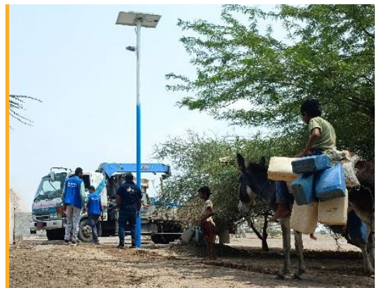
The ETC supported the installation of 35 solar lights in the camp for internally displaced people in Mokha for enhanced safety. Photo: WFP/ETC
