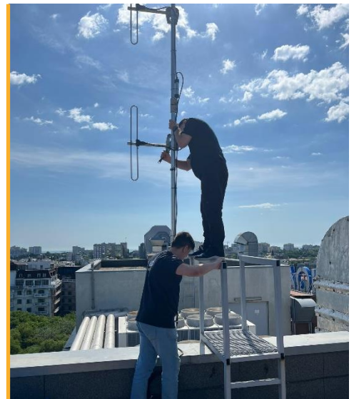
ETC installs equipment on the roof of a new office being used by UN agencies in Kharkiv after relocating due to active shelling. Photo: WFP/ETC
