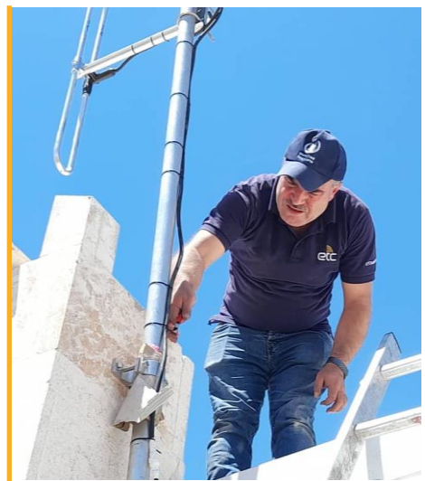
The ETC installs a VHF repeater at the WFP warehouse in Aleppo to enhance secure communications. Photo: WFP/ETC
