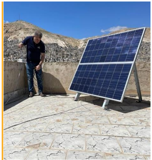
The ETC installs a solar power system in Damascus to ensure uninterrupted power supply. Photo: WFP/ETC
