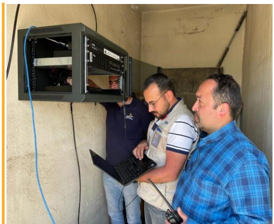
The ETC installs a VHF repeater at the UN hub in Hama to enhance security communication. Photo: WFP/ETC
