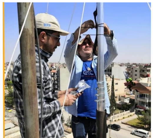
The ETC team upgrades the telecommunications infrastructure at the UN Hub in Qamishli. Photo: WFP/ETC
