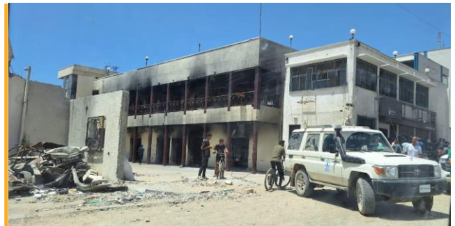
Damage at UNRWA school in Rimal neighbourhood of Gaza City. Photo: UNICEF/ Wondayferam
