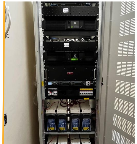
VHF radio repeater site at Al Shaboura Clinic in Rafah is operational 24/7. Photo WFP/Burak Sezgin
