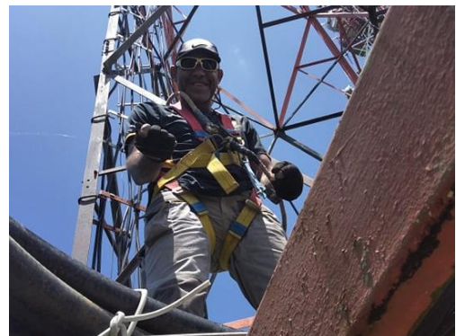
VBTC install telecommunications equipment in Santo to restore radio broadcast services severely impacted by Cyclone Harold.
