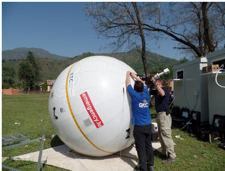
Installing the emergency.lu satellite antenna in Deurali Gorkha District. Photo: WFP/ Mariko Hall
