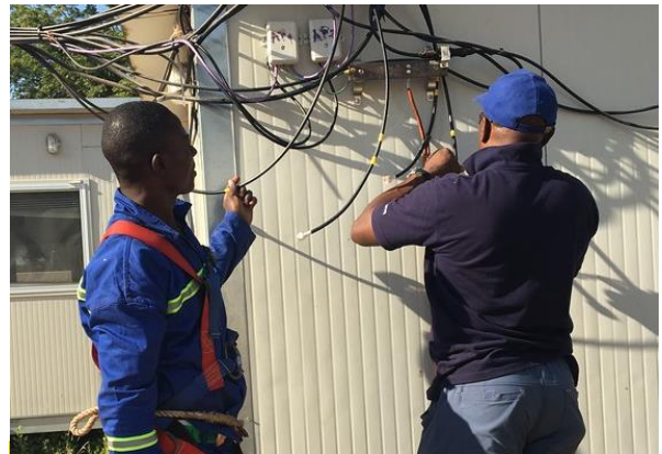
The ETC carries out installations and maintenance at the Security Operations Centre (SOC) in Birao in early 2020.
