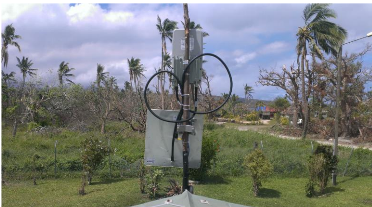
ETC partner Ericsson Response connects local power company, UNELCO, to the ETC network on Tanna. Photo: Ericsson Response/ Michael Duffin
