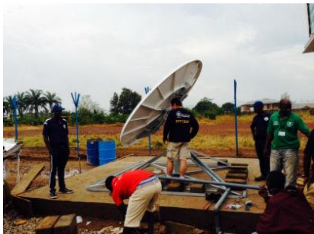
ET Cluster installs a VSAT in Port Loko, Sierra Leone to give 80 humanitarians reliable internet access.
